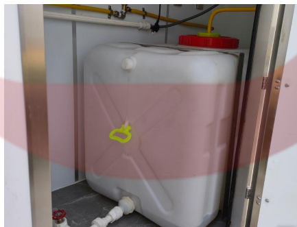
- Clean Water Tank -
