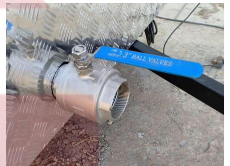
- Holding Tank Outlet -
